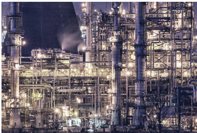
Fig. 1. An example petrochemical processing plant in Grangemouth, Scotland (CC Public Domain, Source: pxhere.com). Oil and gas plants are characterized by a large number of pipes subject to atmospheric and processing elements, causing corrosion.
